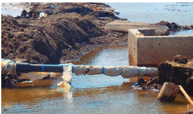
FIG. 3 SRDIP pipe remaining in tact during the 2011 Japan Earthquake
