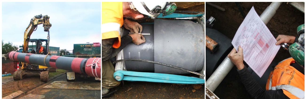
FIG. 9 Typical handling, jointing and workmanship quality checks of DN400 Kurimoto SRDIP installed at Cleat Street Porirua City.
