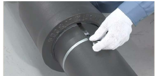
FIG. 8 Quality assurance check with an installed pipe-joint measuring the pipes gasket position to the first witness mark.
